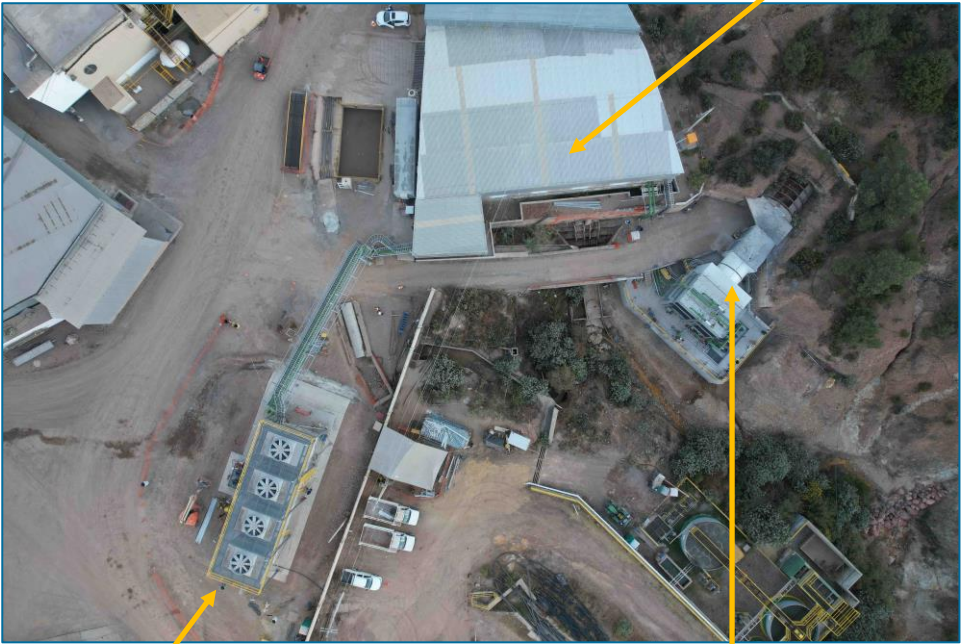
Condenser Cooling Towers
